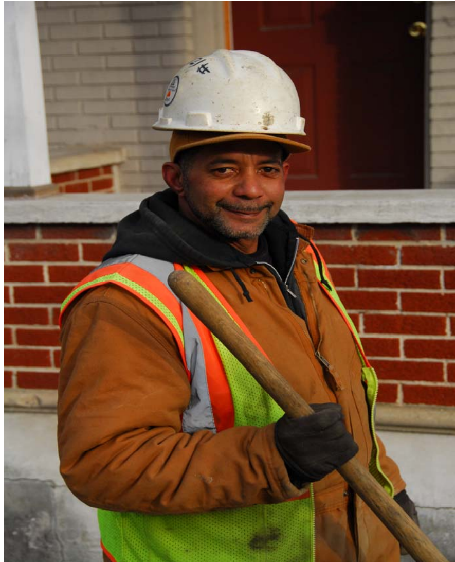
JEFFREY TABRON OF CICCICO CONSTRUCTION WORKS ON A RECOVERY ACT CURB RAMP PROJECT IN OXFORD, CHESTER COUNTY.
